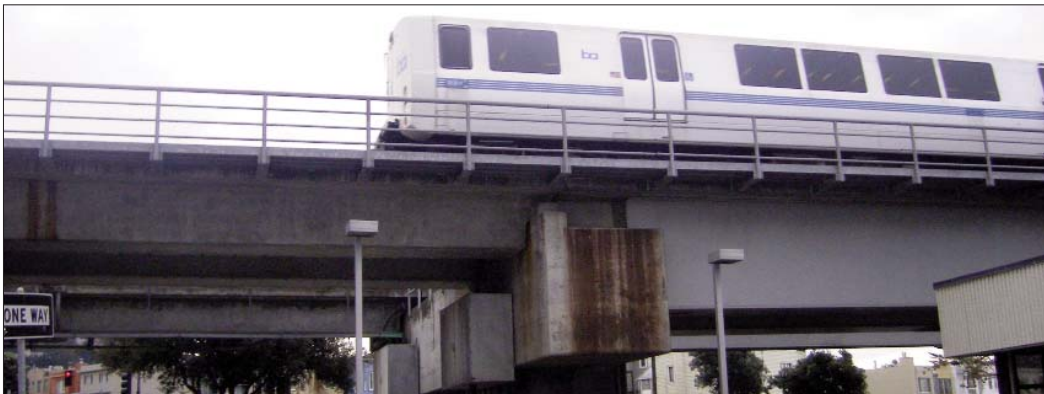
The column in the center of the photo, and the dark colored beam to its left, are part of the original elevated structure at Daly City. The lighter colored beam to the right of the column is part of the new extension over John Daly Blvd.
